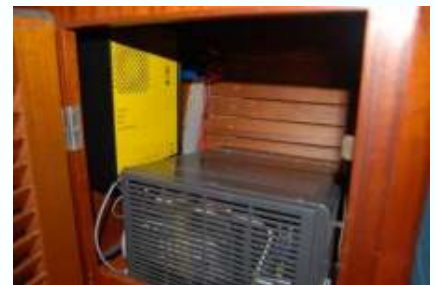
24v/220v Charger/inverter and 12v charger
